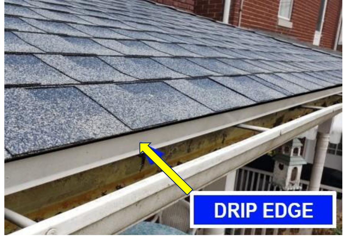
Drip Edge Moldings on All Edges of Roof Where Water Flows Into Gutters
